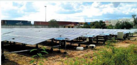
In 2016-17, 200 KWP of Solar Plant was installed at Manali, Chennai which is capable of generating 27000 units of power per month and offsetting around 300 tons of carbon dioxide each year. This plant will supply power to the Greases & Lubricants, Industrial Packaging and Leather Chemicals manufacturing units at Chennai.
